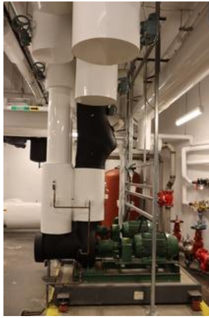
Part of the complex plumping
