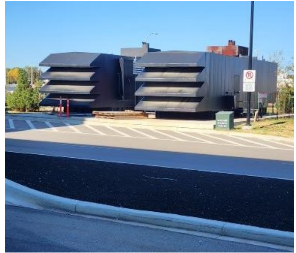
These are the massive generators that are available if a power outage is experienced.
