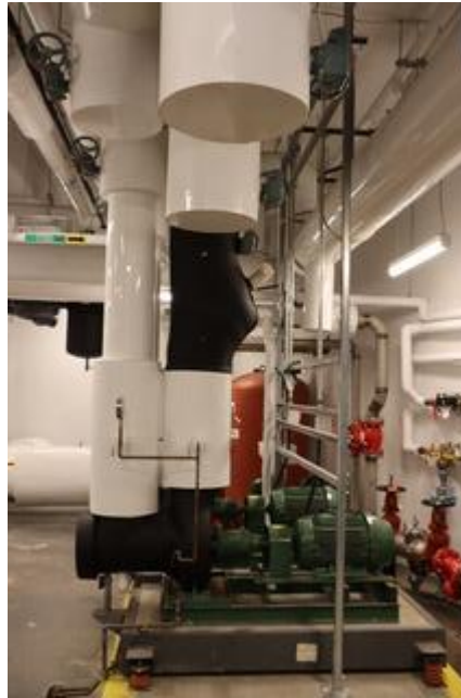
Part of the complex plumbing
